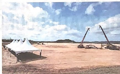
Tents have been set up at the Kedah Rubber City project site.
