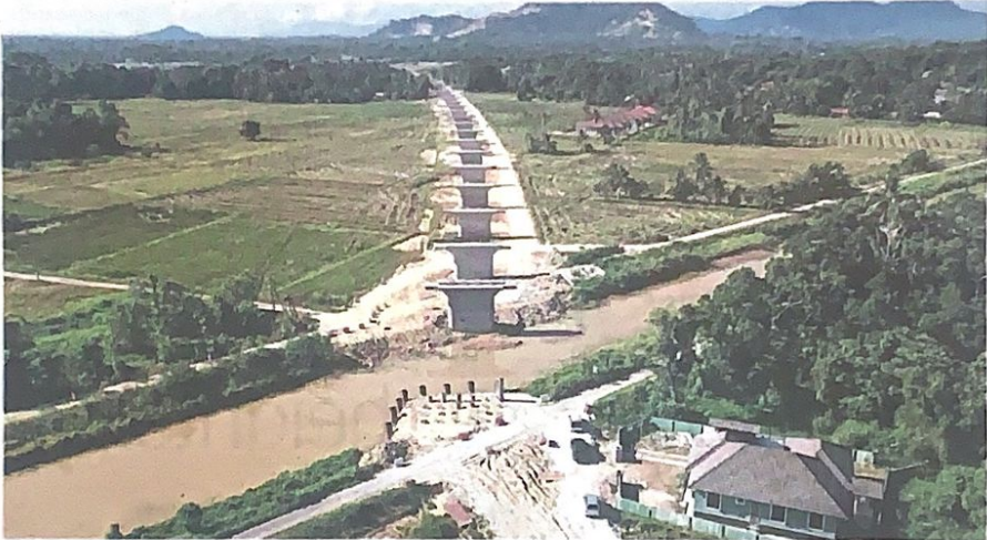
Coming up: Construction work on the alignment of the ECRL being carried out in Kampung Padang Lengkuas, Padang Pisang in Kota Baru. — Bernama
