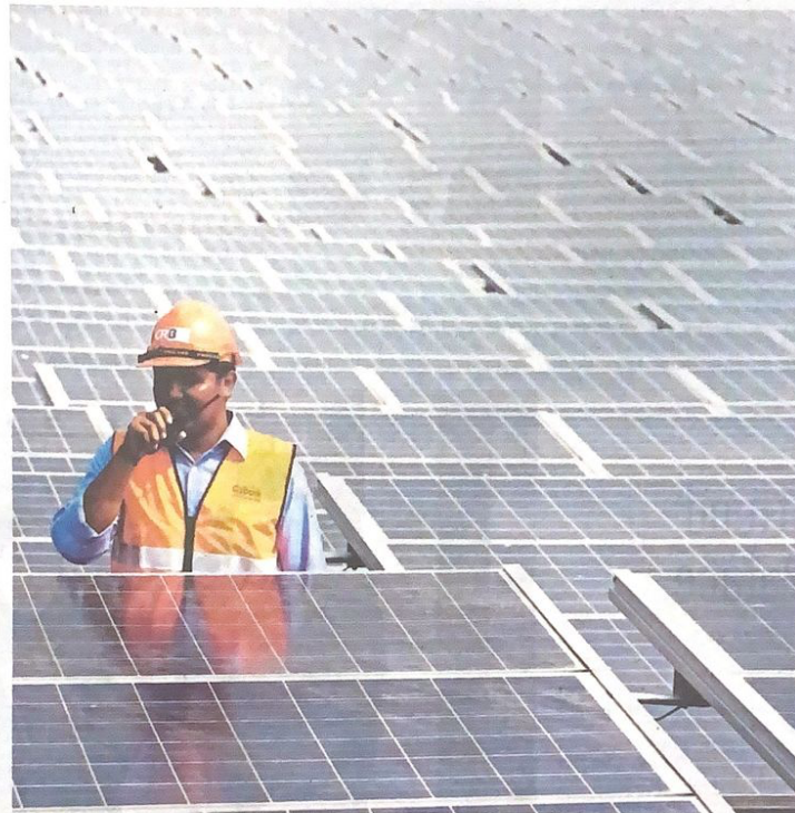
A solar energy farm in Seremban. Backed by 12 strategies and 31 action plans, the National Energy Policy 2022-2040 will open a new chapter in the country's energy sector. FILE PIC
