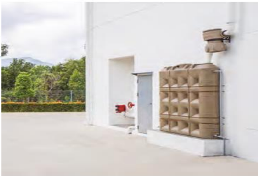
Figure 7.6 Rainwater Harvesting Tank at i-Park's Factories
