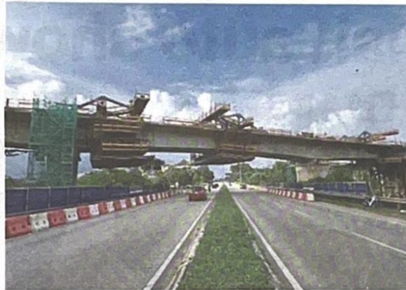
Fits like a puzzle: ECRL's Kuantan Bridge was successfully constructed across Jalan Kuantan-Sungai Lembing.
