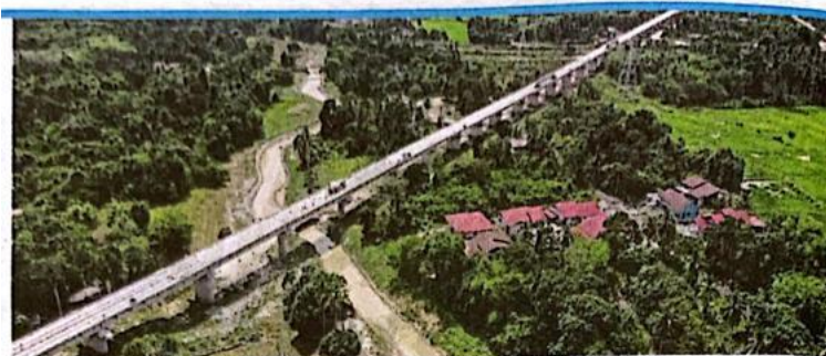
Beams being installed on the East Coast Rail Link in Bachok yesterday. BERNAMA PIC
